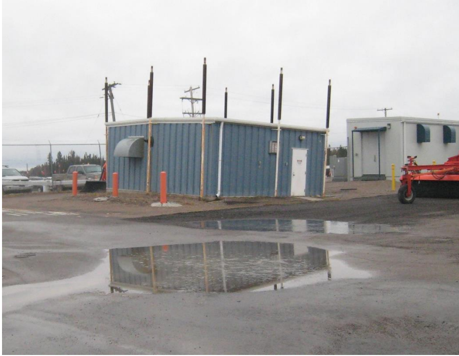
Figure 5. Severe tilting of a maintenance building due to permafrost degradation.
