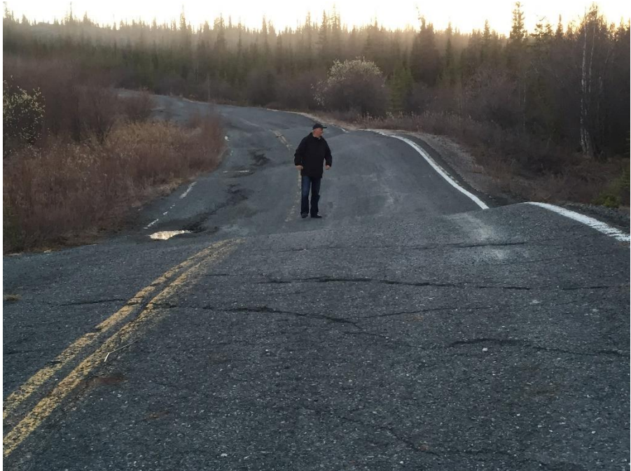
Figure 6. High severity pavement deformations on a road in the Yellowknife Area.
