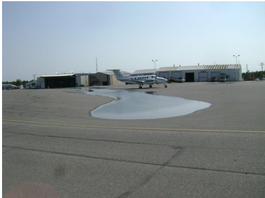
Figure 4. Water ponding in a deep depression on apron pavement at Thompson Airport.
