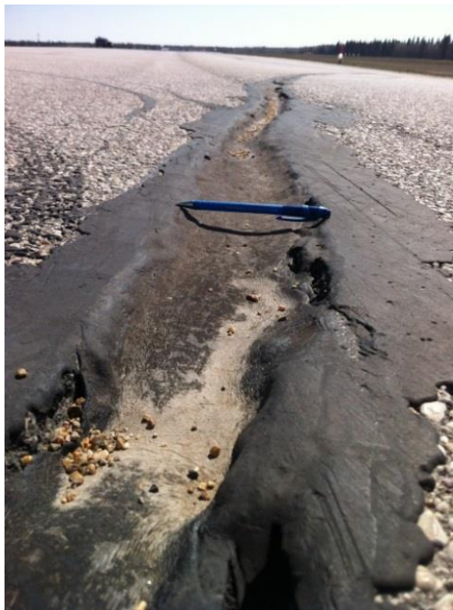
Figure 2. Severe transverse crack on runway at Hay River Airport.
