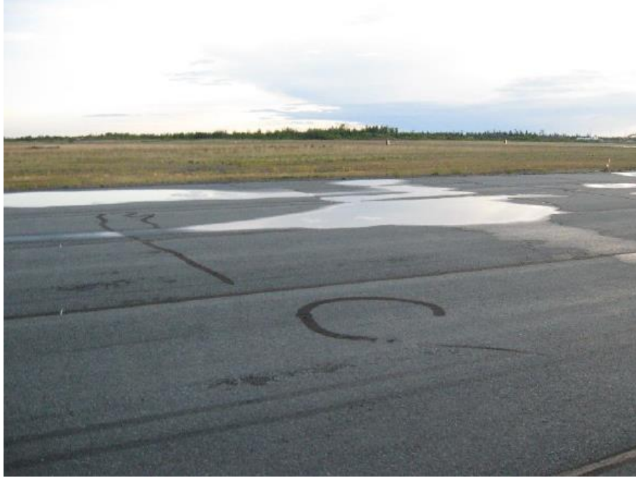
Figure 3. Water ponding in a deep depression on runway pavement at Yellowknife Airport.
