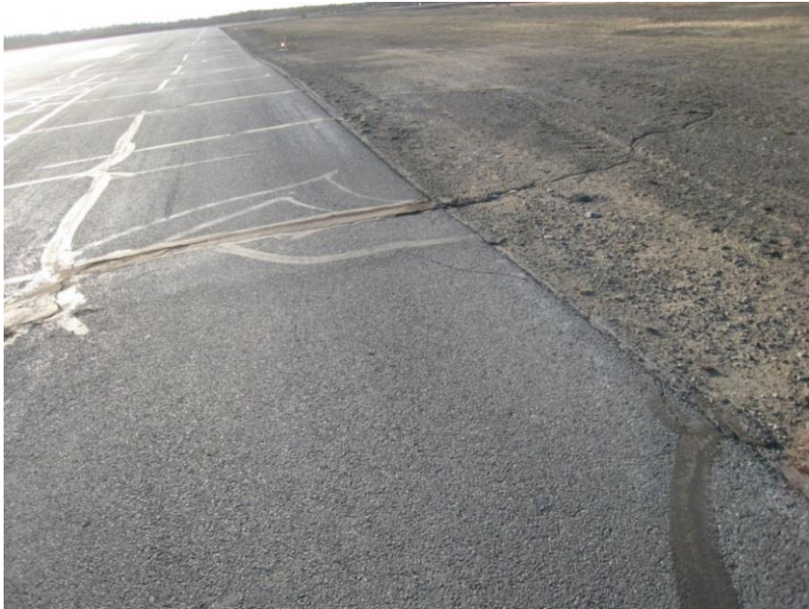
Figure 1. Severe settlements in the non-keel zone of runway pavement at Yellowknife Airport and cracking in granular shoulder.
