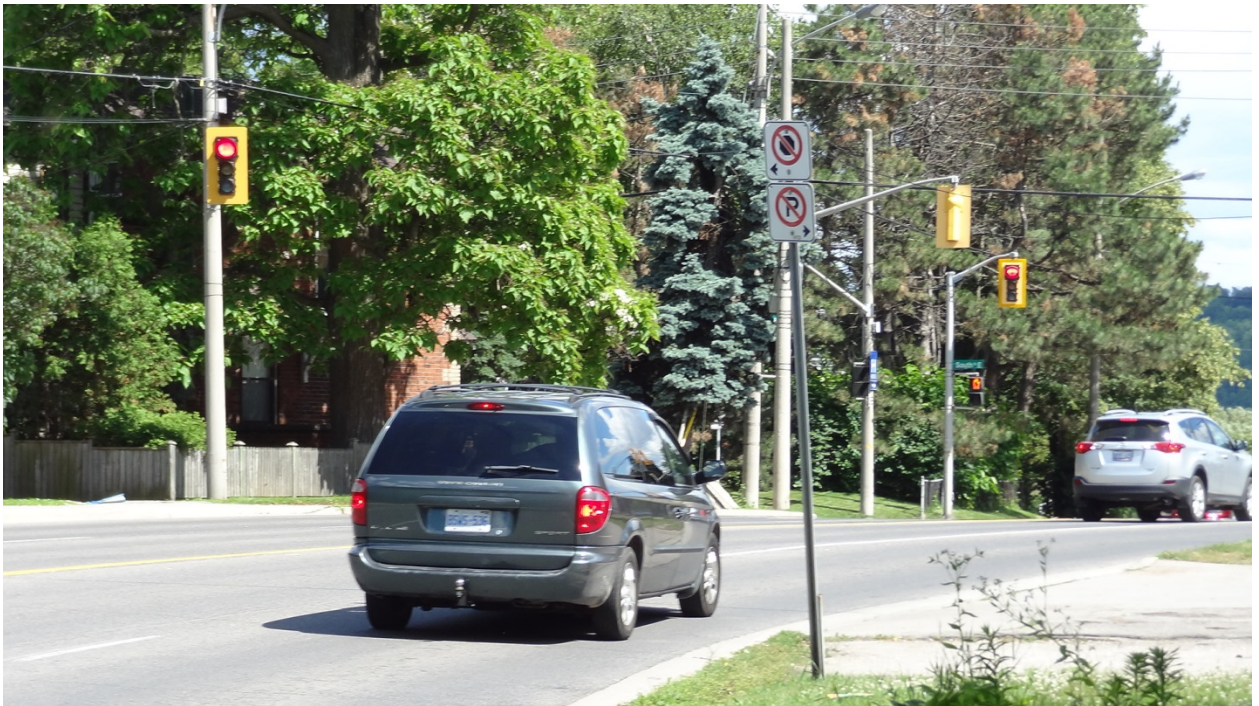
Figure 3. Use of Auxiliary Traffic Signal on Sharp Horizontal to Improve Signal Conspicuity and Driver Compliance
