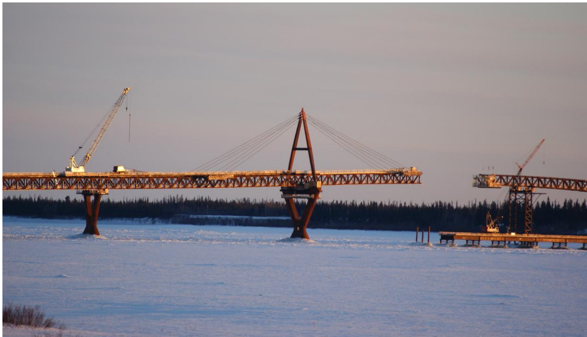
Fig. 5: Piers 3N and 4N with temporary works during winter 2011/2012 (Photo: Arndt Becker, Infinity)
