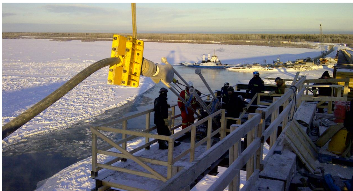
Fig. 11: Cable installation with ferry “Merv Hardie” in the background (Photo: Chad Amiel, Infinity)
