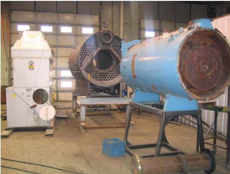
Economizer, Main Boiler and Air Coil
