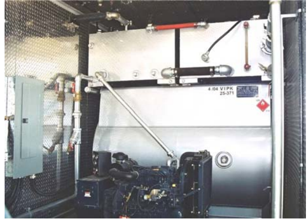
Holding Tank, Fuel Tank, and Generator
