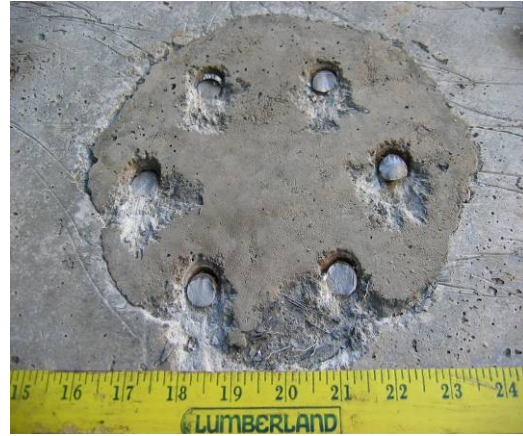
Figure 9 Grout pocket damage
