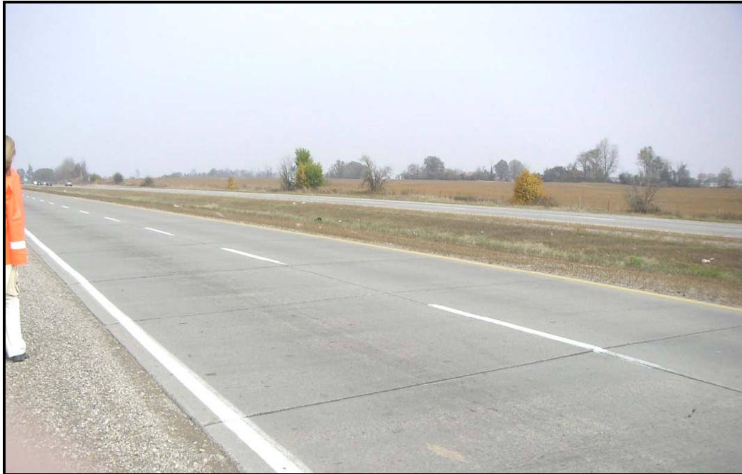
Figure 4. Typical Condition of Unbonded Concrete Overlay, SBL
