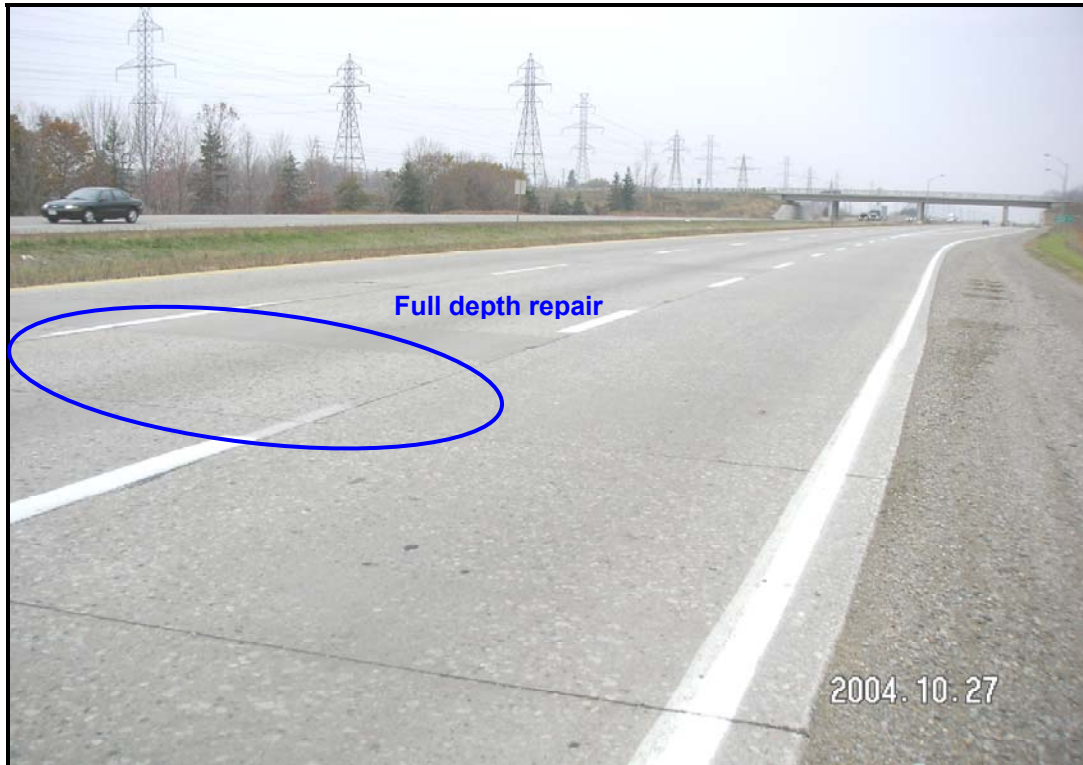
Figure 3. Typical NBL Pavement Condition
