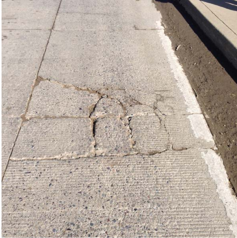
Figure 6 – April 2015 photo of BCO failed panel in outer turning lane
