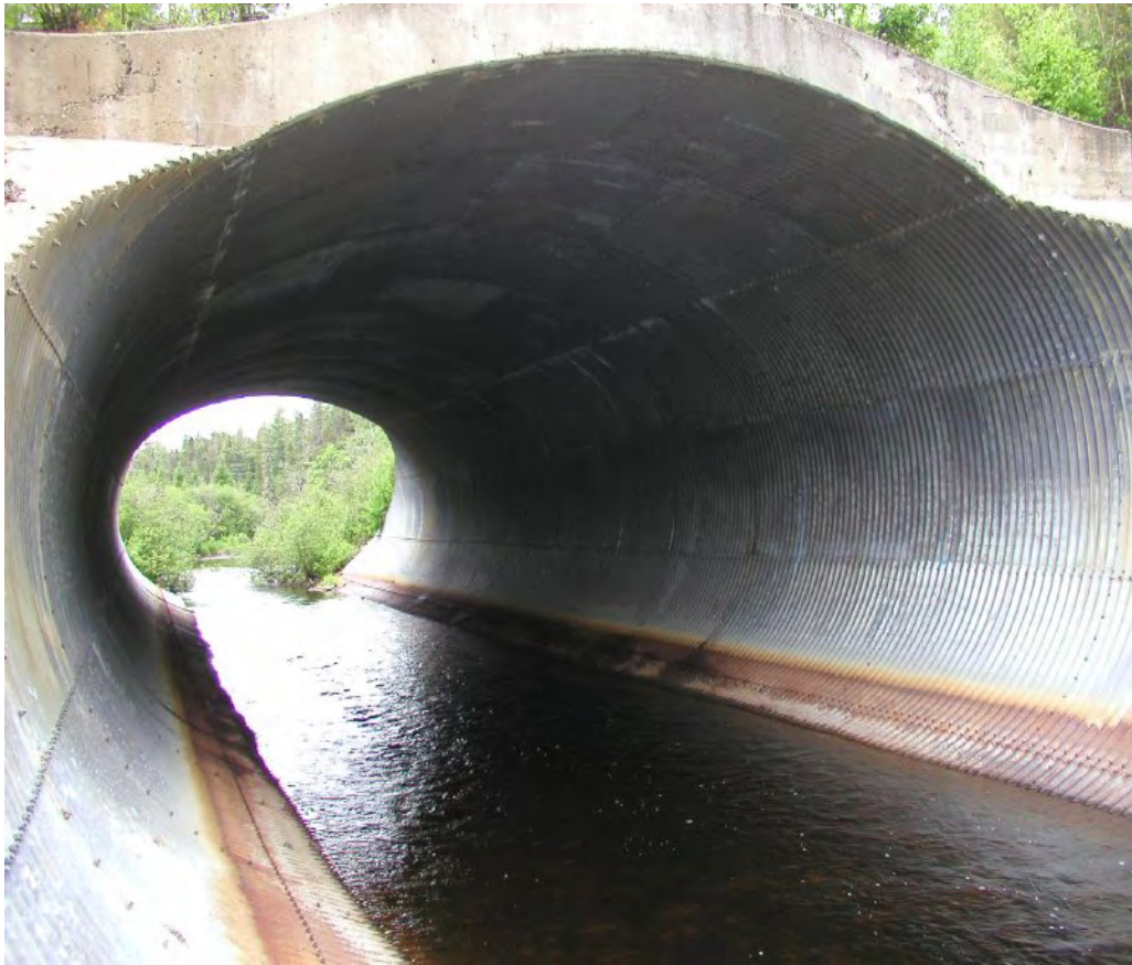
Figure 1: Typical SPCSP Bridge Showing Rust in Lower Quadrant
