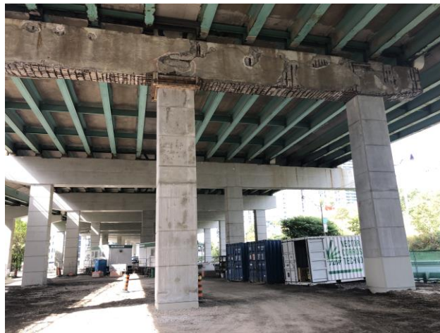
Figure 14. Completed Piers in the Background with a Partially Completed Pier in the Foreground
