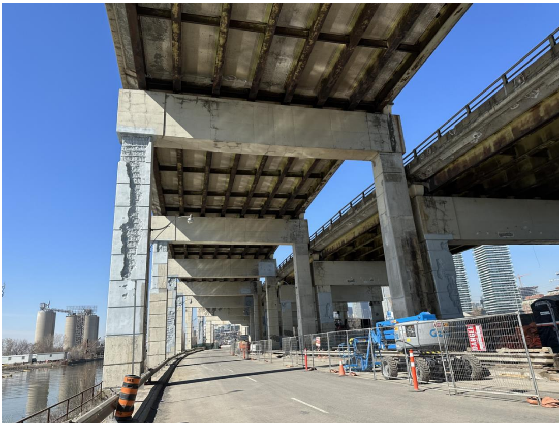
Figure 17. Spalled and surrounding areas protected with ASZ+ anodes
