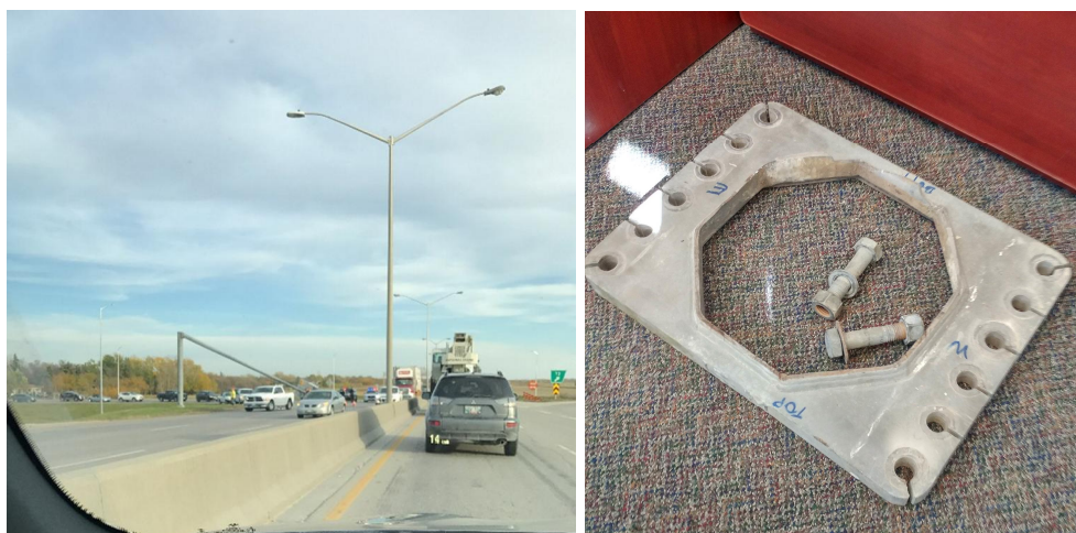
Figure 2: Failure of Cantilevered Structure as a Result of Fatigue (Left) and Failure Location at Arm/Flange Connection (Right)
