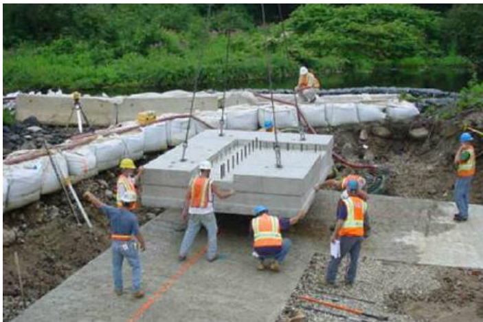
Figure 3: Placing the precast footing on the sub-footing. The sub-footing does not need to be formed. (Source: PCI)
