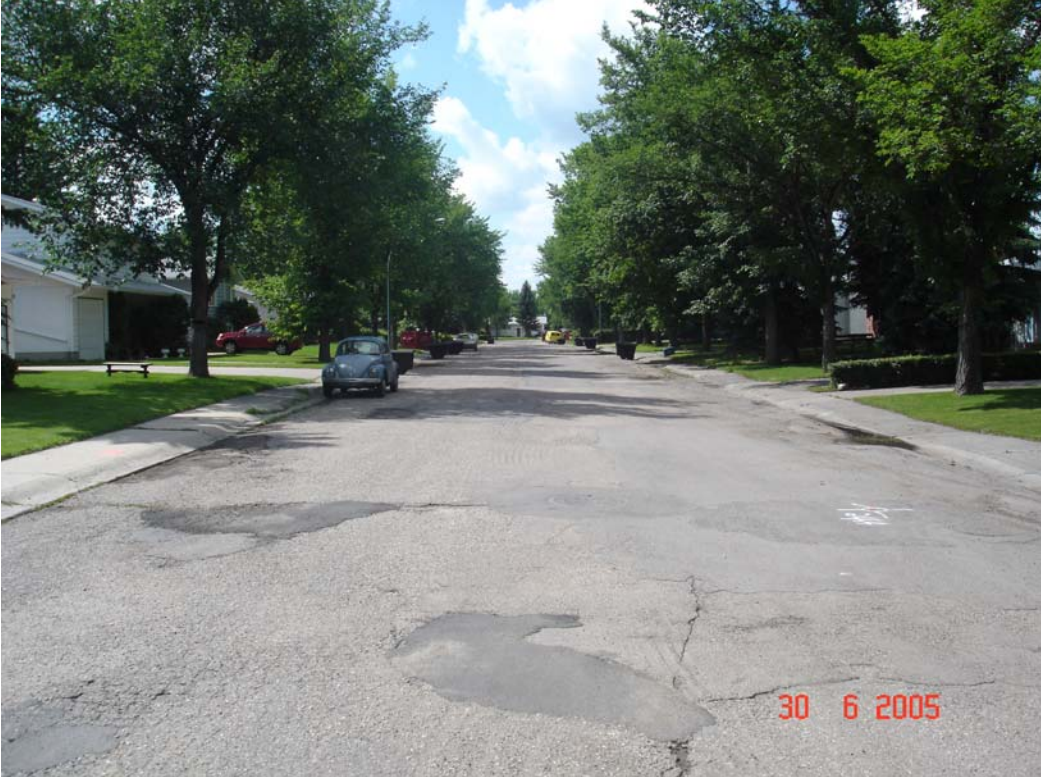
Figure 1 Typical A Priori Surface Distresses of Shannon Road
