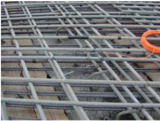
(c) Fiber optic sensors on FRP bars and embedded in concrete (Wotton Bridge)
