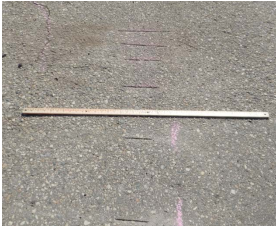
Figure 10: Testing the Minimum Crack Length
