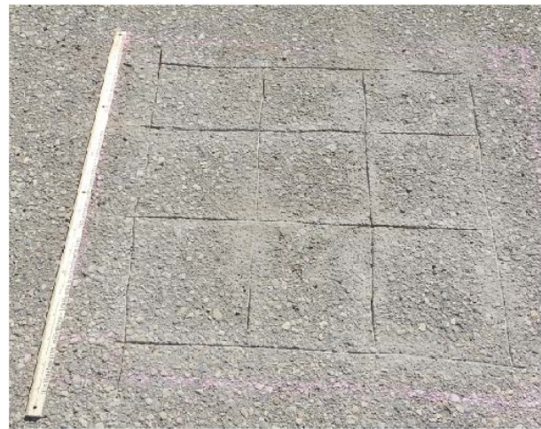
Figure 13: Saw Cut Non-Wheel Path Block Cracking
