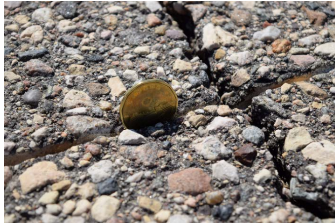
Figure 11: Saw Cut Crack Width
