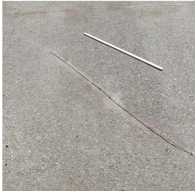
Figure 9: Saw Cut Meandering Crack
