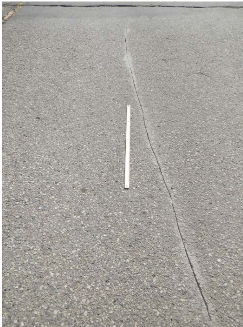
Figure 8: Saw Cut Longitudinal Crack
