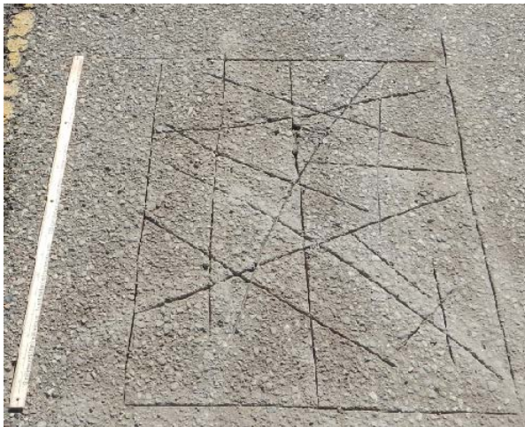
Figure 12: Saw Cut Wheel Path Block Cracking
