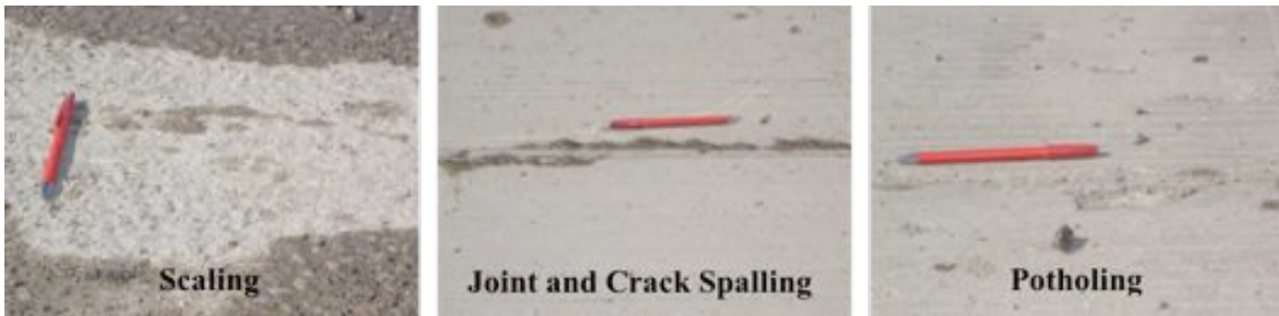
Figure 7. Test Section PCI Photos – Apr. 2, 2008
