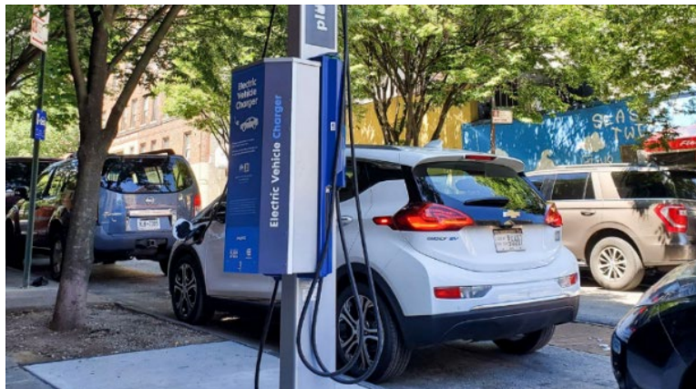
Figure 2-29: Curbside EV Charging Station
