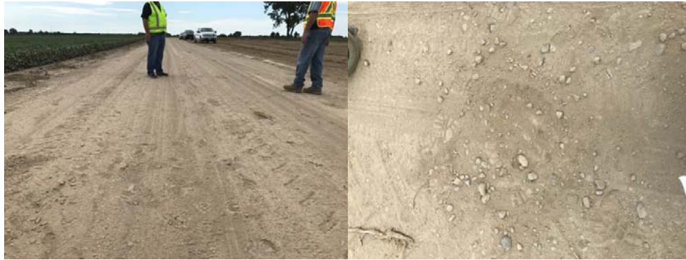
Figure 5. Gravel loss of surface in T41, pictures taken in July, 2018
