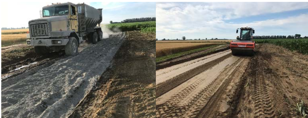
Figure 1. Pictures showing the stabilization. Cement spreading (left); compaction using sheep's foot roller (right)
