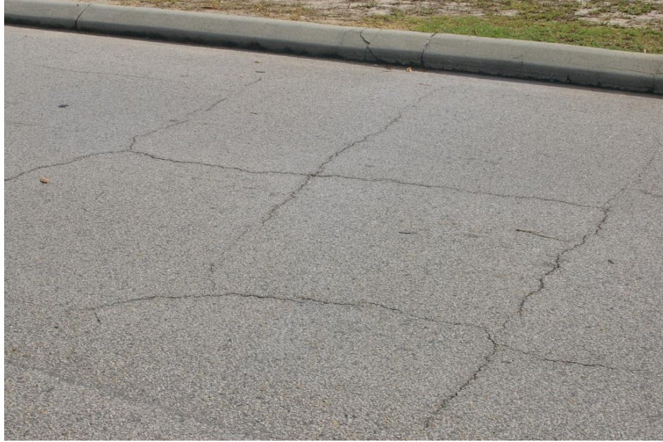
Figure 3: Block cracking in asphalt pavement
