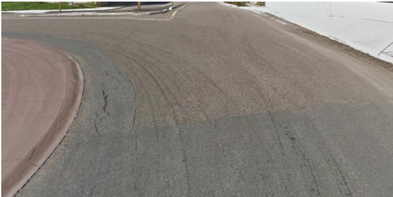
Figure 2. Example of distresses of asphalt pavement at roundabouts.
