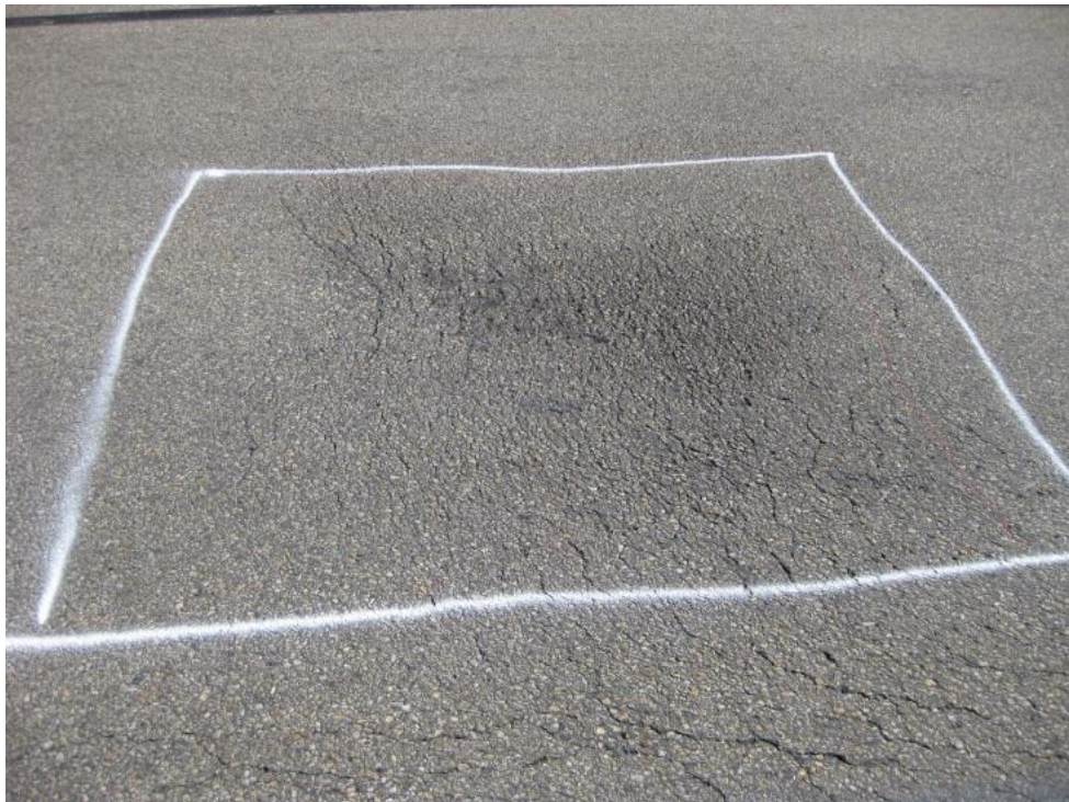
Figure 6. Example of airfield asphalt pavement severe shoving.
