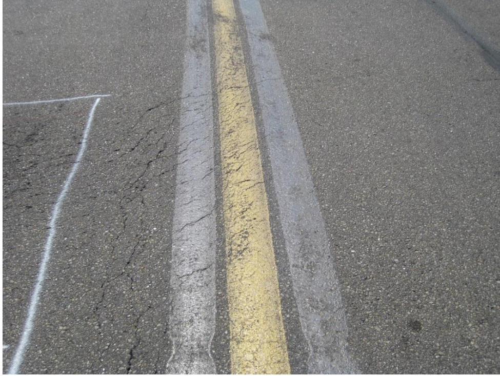
Figure 5. Example of airfield pavement shoving, cracking and slippage.
