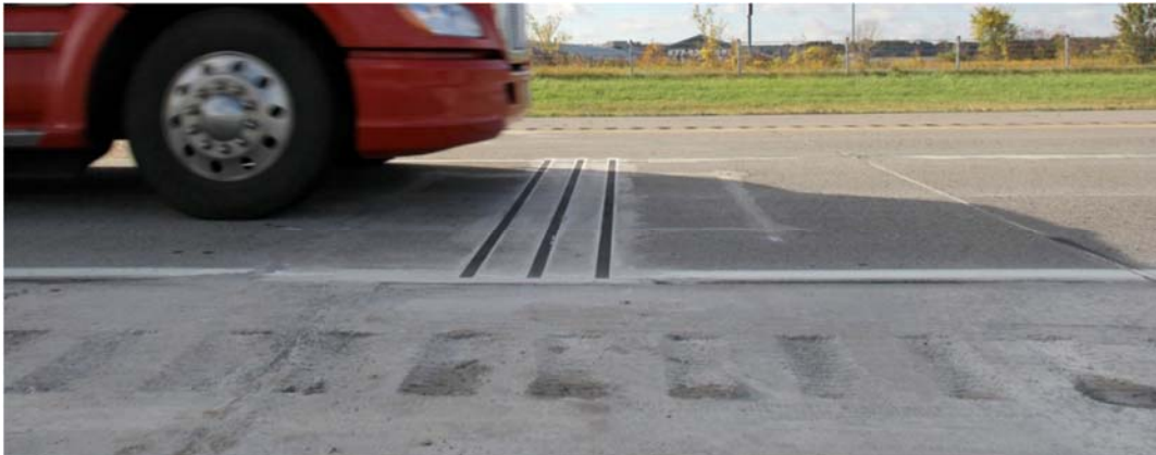
Figure 2 IRD VectorSense™ Sensors Installed on Road
