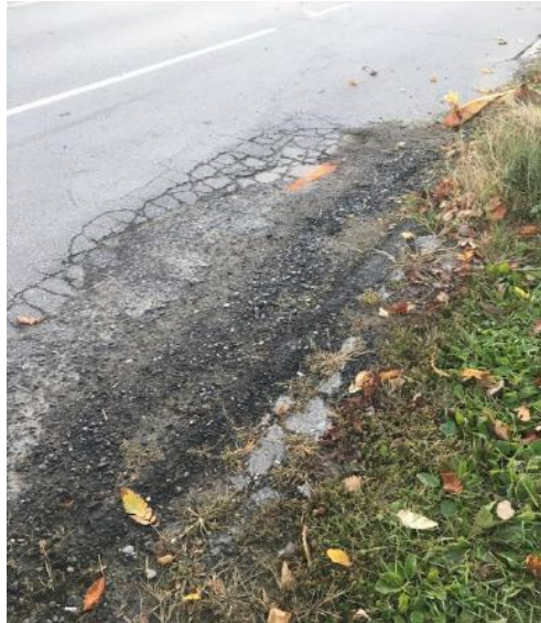
Figure 1: Distress at Bus stop
