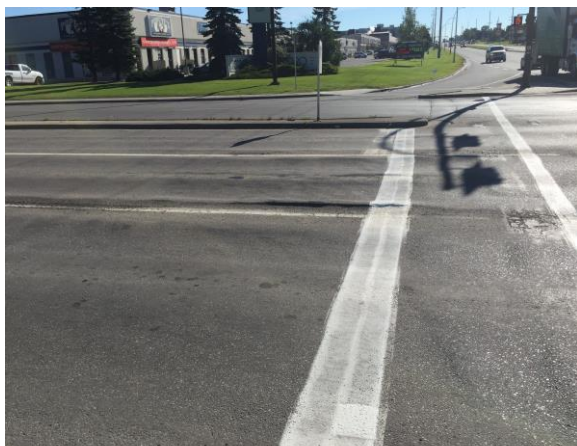
Photo 1: Instability rutting at the approaches to an intersection
