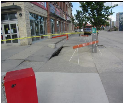
Photo 3: Undermined Sidewalk affected by 2013 Floods
