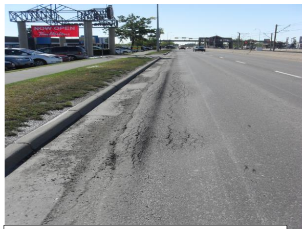
Photo 2: Instability rutting caused by the Transit buses at approaches to a Bus Stop
