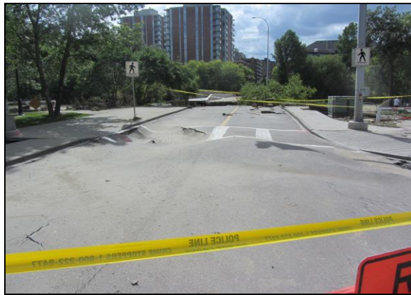
Photo 4: Roadway segment damaged by 2013 Floods
