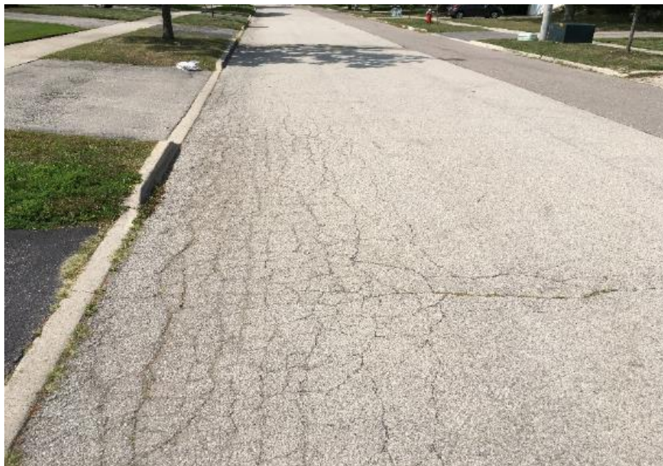
Photo 1: Pavement Edge Alligator Cracking – Frankfield Ave
