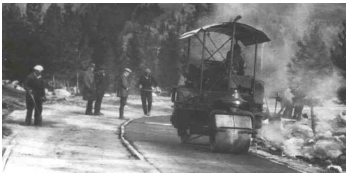
First commercial paving with bituminous sand in Jasper, Alberta, 1926 (Source: Public Archives of Canada)
